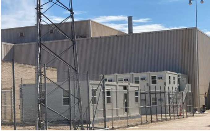
WillScot Mobile Mini prepared 83 FLEX units and 12 modular offices in a safe and timely manner for a 62-day nuclear plant shutdown for maintenance in St. Francisville, LA.
