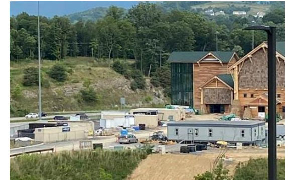
Storage containers, ground-level offices, mobile offices and job site services being used during a Bass Pro Shop remodel in Morgantown, WV.
