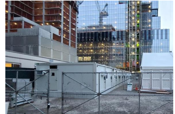
The second of five COVID-19 testing and vaccination facilities for One Medical located at Hudson Yards, NY.
